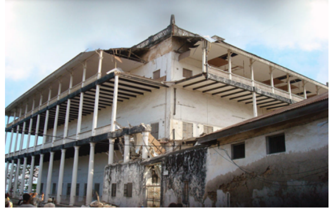
Figure 2: A corner section of the House of Wonders that collapsed in November 2012 (Source: WMF 2017)
